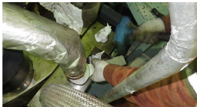
Unauthorised tightening by means of a wrench and a hammer
